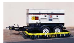
Portable Generator Containment
