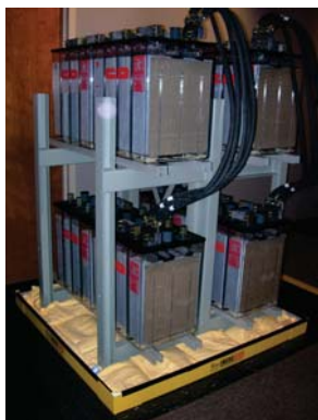
Eagle Modular UL Spill Containment
